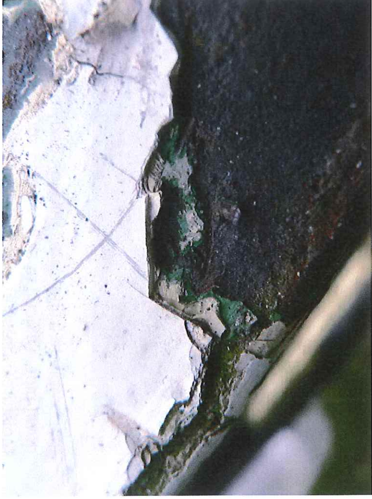
Handrail paint layers in close up. Evidence of early Green layers under cream and white coats.
